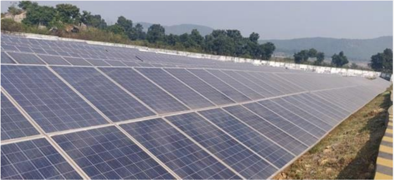
Figure 1 Ground Mounted Solar panels in MCL
